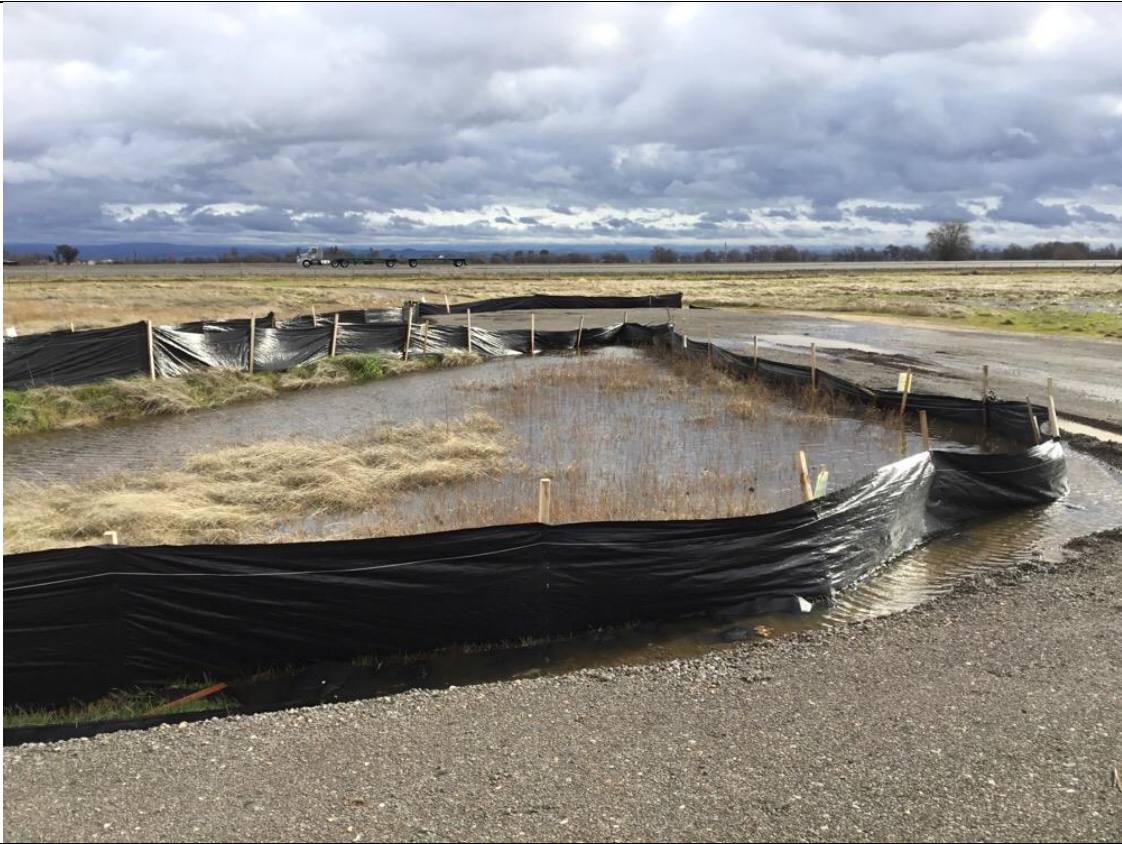
Photo 5: Vernal pool feature at Pull Site 0/1B was inundated due to wet weather. Installed BMPs were intact and no adverse impacts occurred because work in the area has already been completed.
